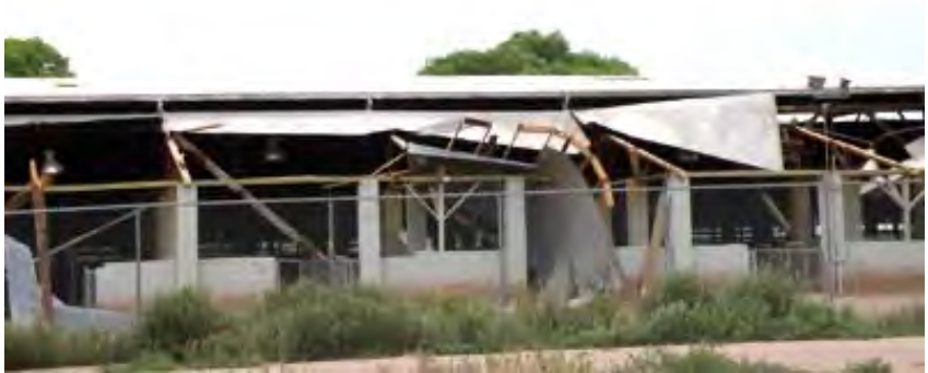
Wind damage, County Fairgrounds, 2012
